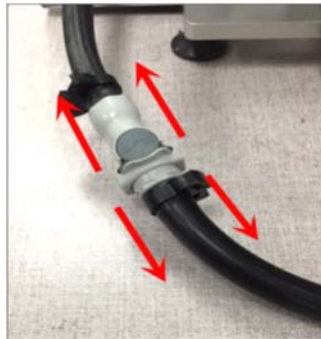
Heater inlet to waterbath
